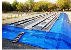
Training Line with Slab Track for Mumbai-Ahmedabad High-Speed Railway
