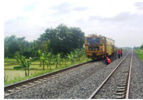
Railway Double Tracking of Cikampek - Cirebon on Java North Line (II), Segment III
