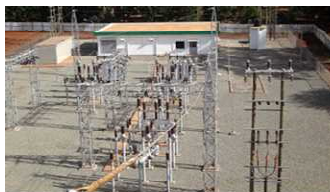
The Project for Rehabilitation of Substation and Transmission Line in Kilimanjaro Region (Tanzania)
