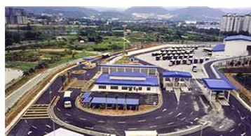
Design, Construction, Completion and Commissioning of Solid Waste Transfer Station at Taman Beringin, Kuala Lumpur (Malaysia)
