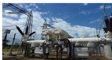
The Project for Improvement of Queensway Substation (Uganda)
